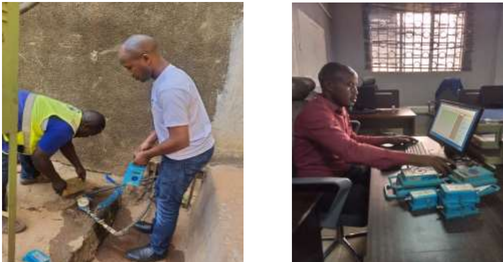
Figure 3.3: Installation of the pressure data logger at customers' meter and downloading pressure data.
