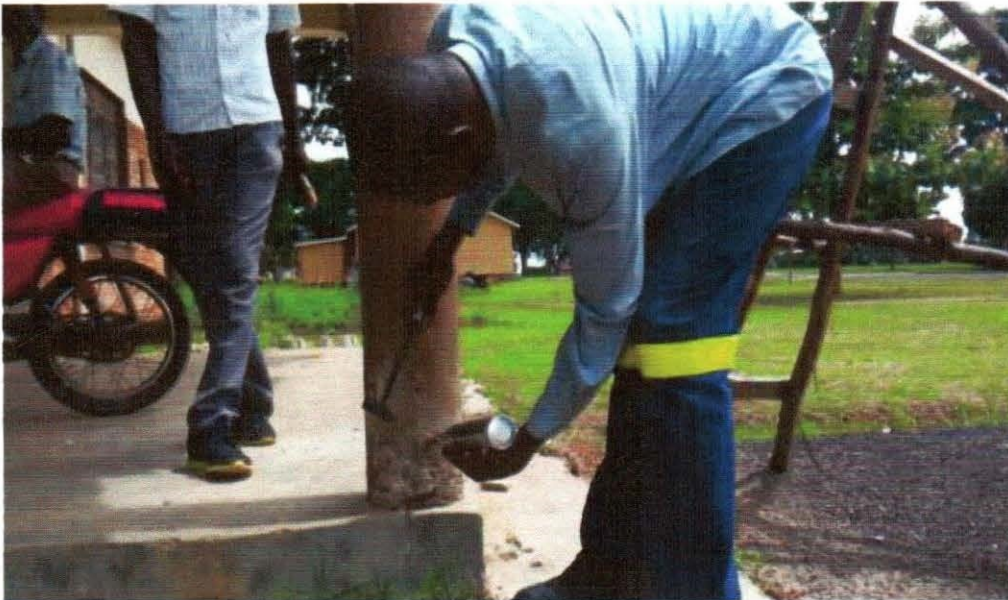
Figure 7.10: Cracks at the bottom of the Column at the District Health Drug Store.
