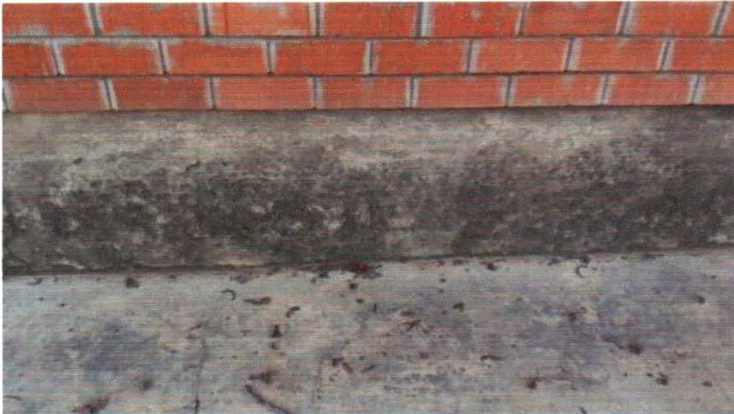
Figure 7.8: Dampness at the External wall of the District Health Drug Store
