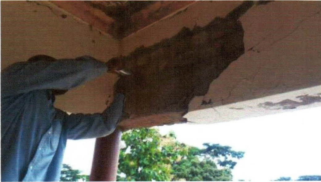
Figure 7.9: Cracked beam at the District Drug Store.
