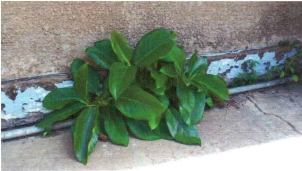
Figure 7.5: Plant growth at the External wall of the Operating Theatre at Amuria H/C IV.
