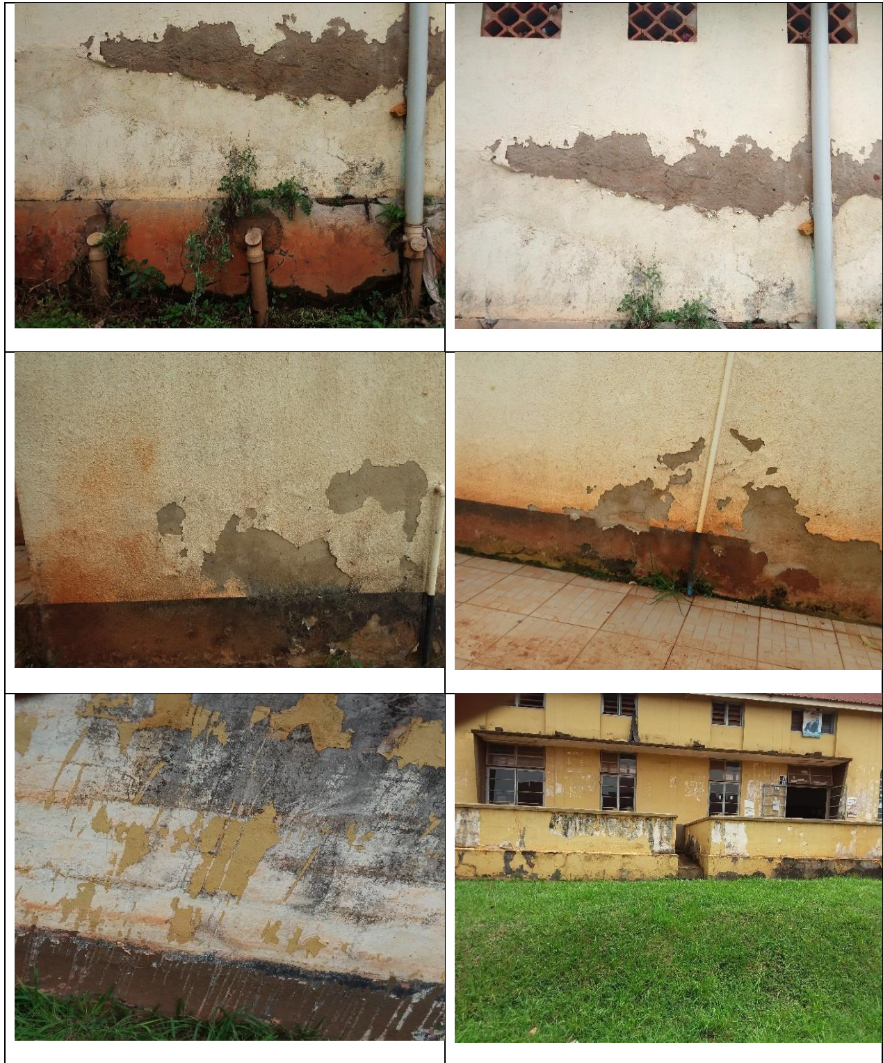
Figure A3.1: Defects in different structures in Kyambogo University - Kampala
