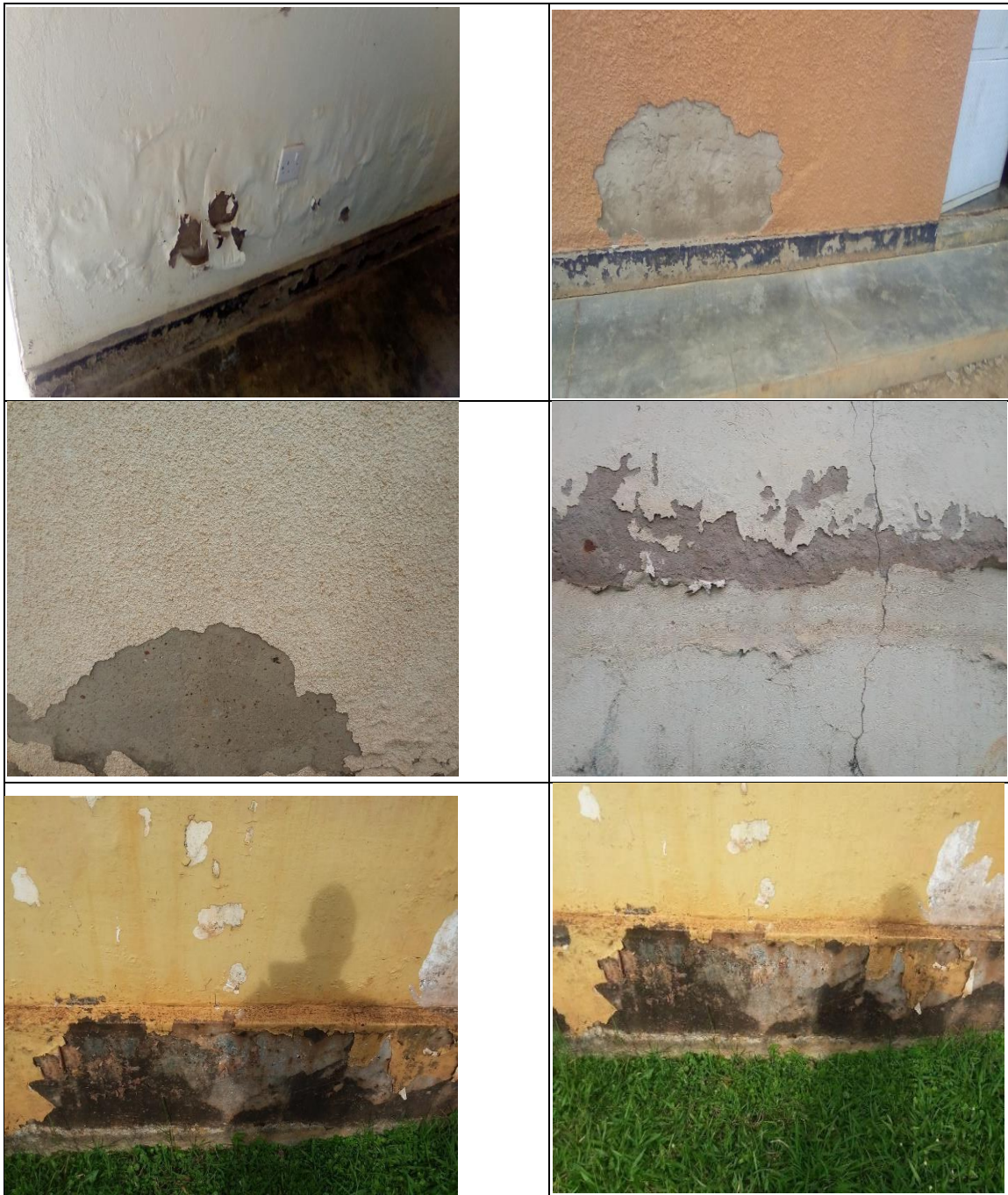
Figure 1.1: Defects in masonry walls
