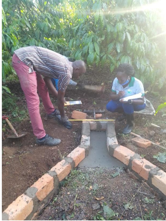
Figure 33: Construction of the runoff trap at Kaweri Coffee Plantation Limited (KCPL), Mubende, Uganda (Source: Author)
