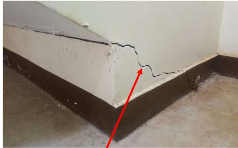
Cracks on the walls
