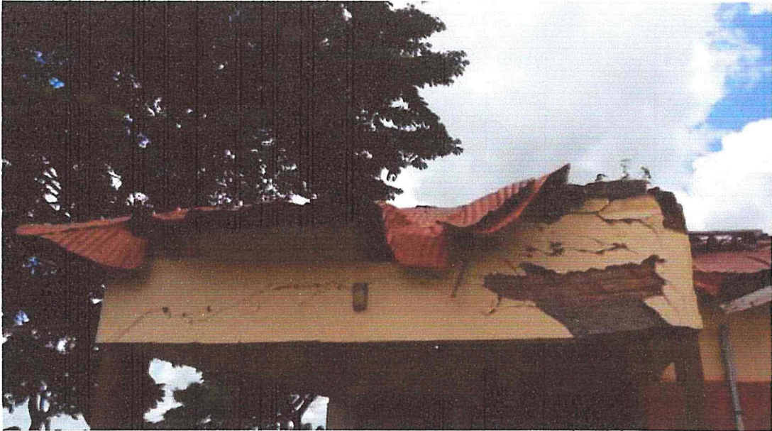
Figure 7.13: Damaged roof structure of Amuria District Health Drug Store
