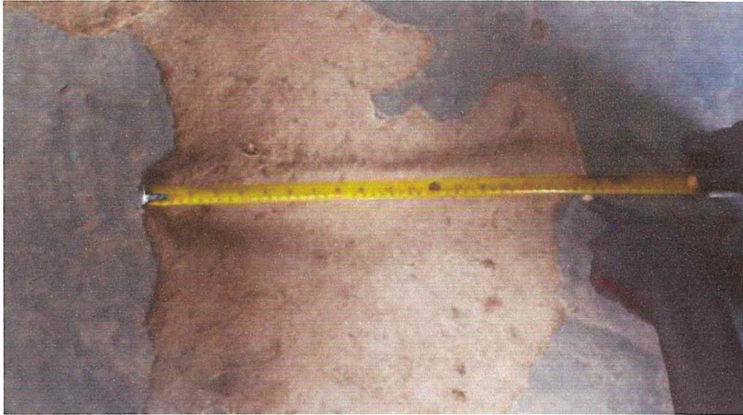
Figure 7.1. Patches on the Council Chambers Cement Sand Screed Floor Finish
