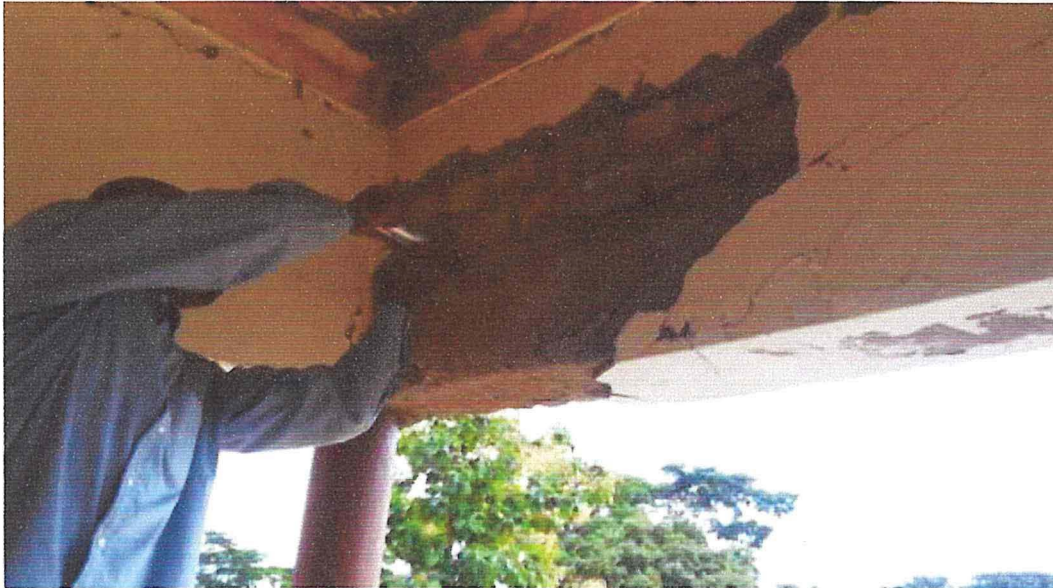
Figure 7.9: Cracked beam at the District Drug Store.
