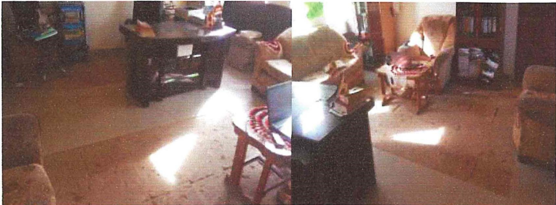
Figure 7.2. Patches of missing Floor tiles at the District Water Office
