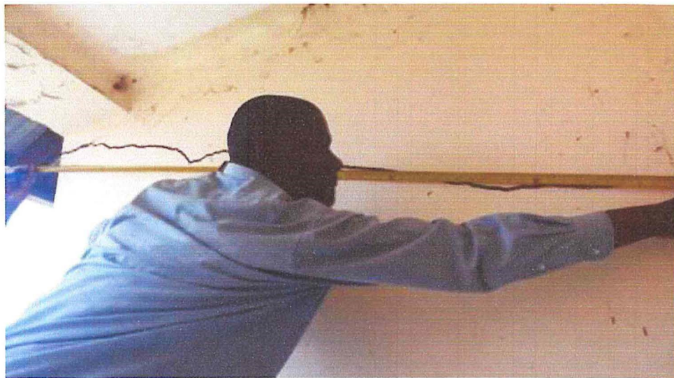
Figure 7.4: Crack along the partition wall of a theatre at Amuria H/C IV.
