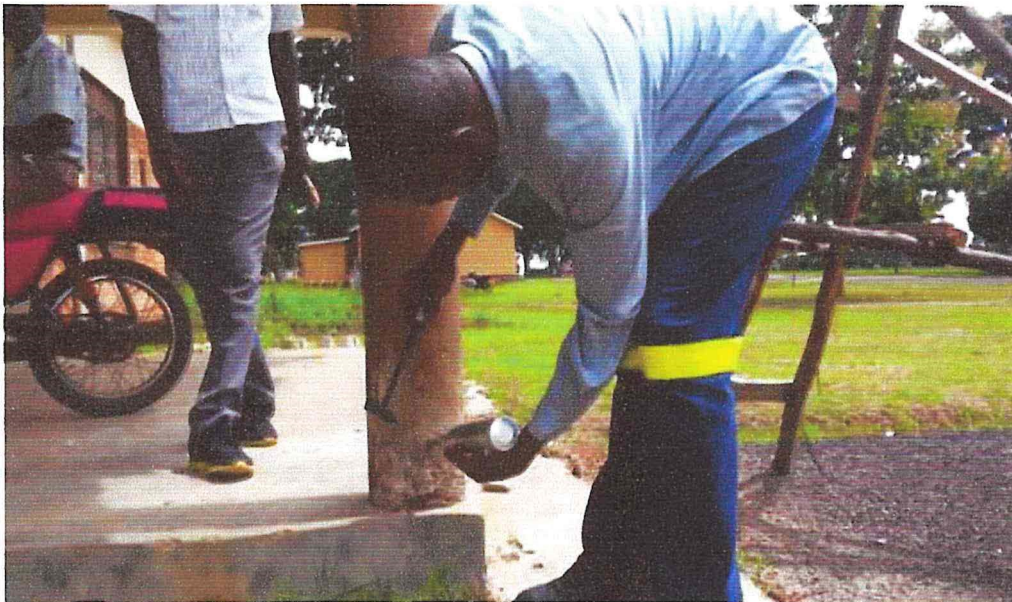
Figure 7.10: Cracks at the bottom of the Column at the District Health Drug Store.
