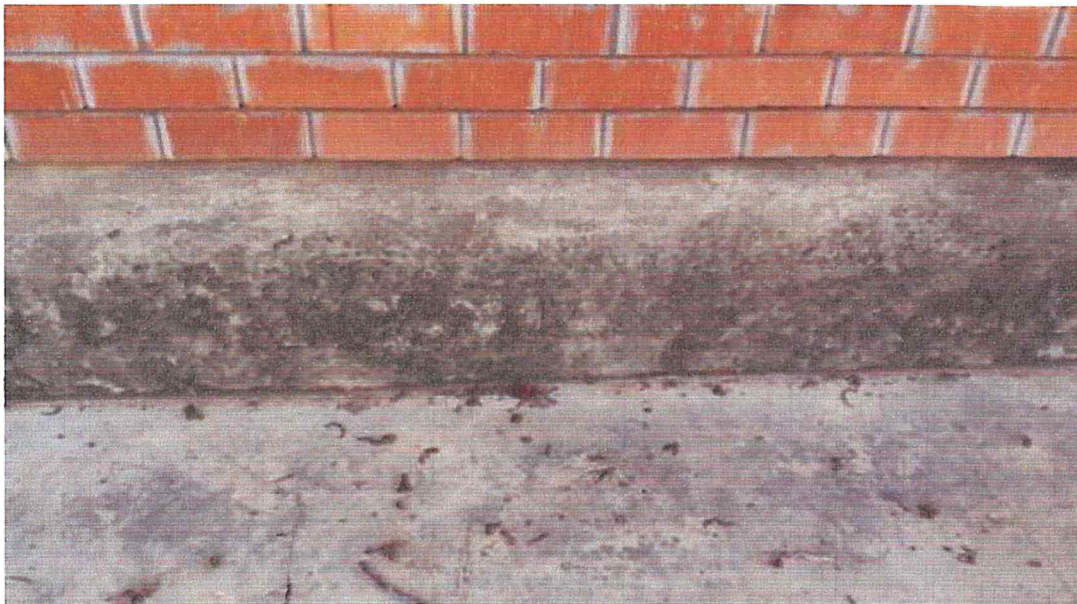
Figure 7.8: Dampness at the External wall of the District Health Drug Store
