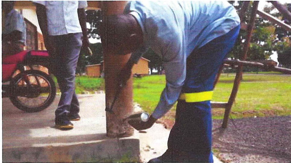
Figure 7.3: Cracks at the bottom of the Column at the District Health Drug Store.
