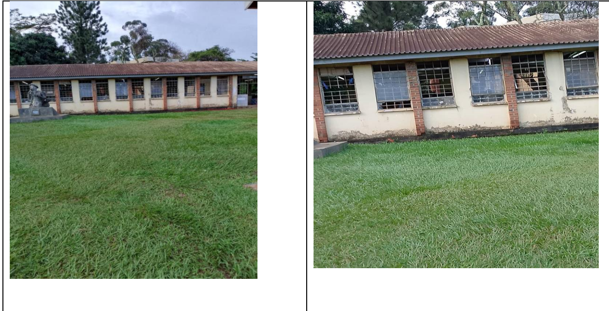
Figure 3: Dilapidated lecture rooms with asbestos roof in KYU
