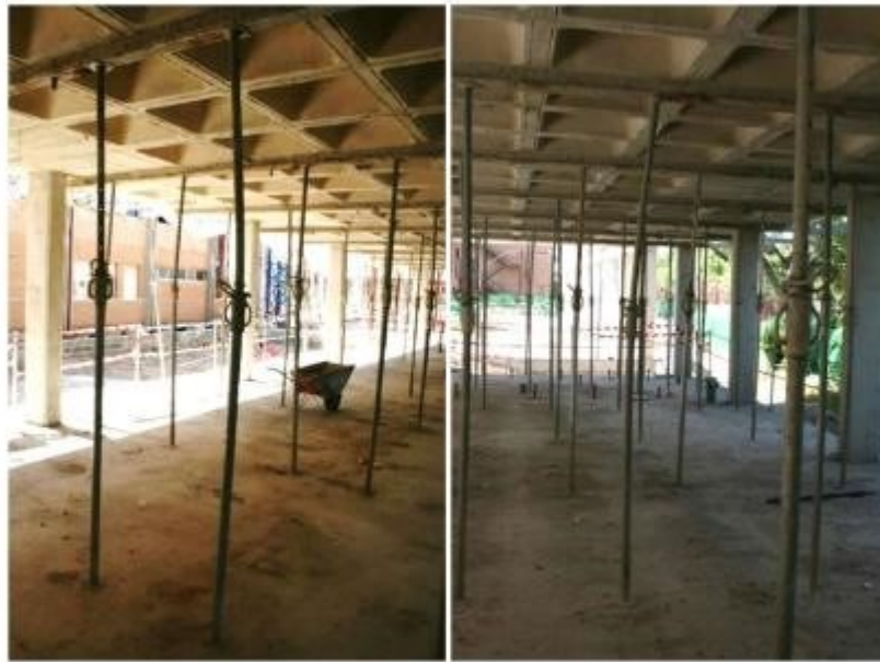
Figure 2.2: (a) Buckling of shores during construction stage (b) Using Load Limiters
