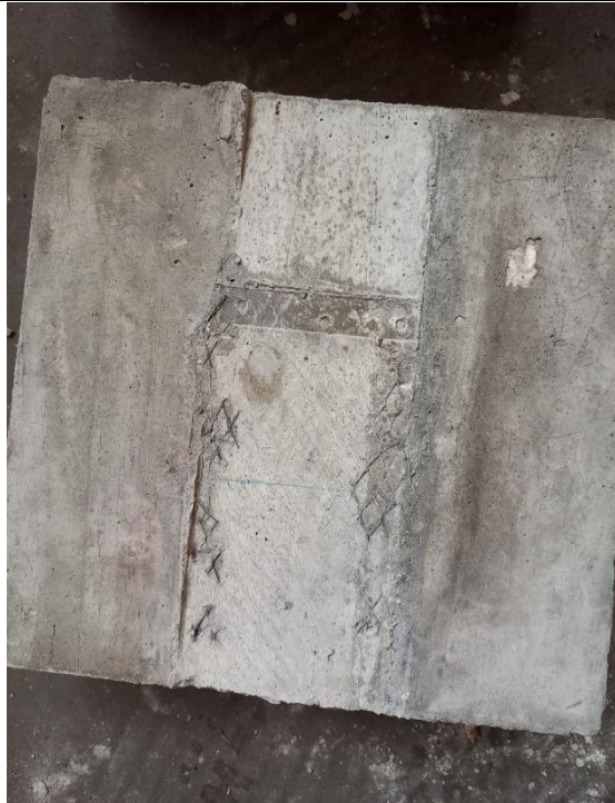
Figure 4.40: Raptured Expanded Metal lathe (Mesh) sticking out of the concrete block
