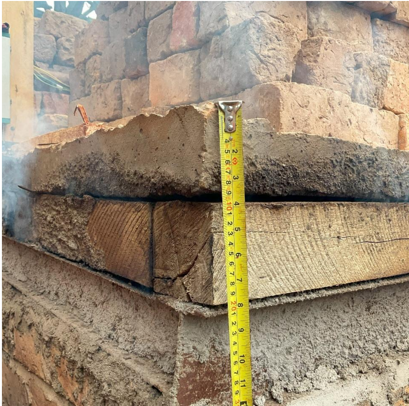
Figure 4.8: Curling at the corner edges of concrete due to expansion caused by temperature rise at the bottom of concrete
