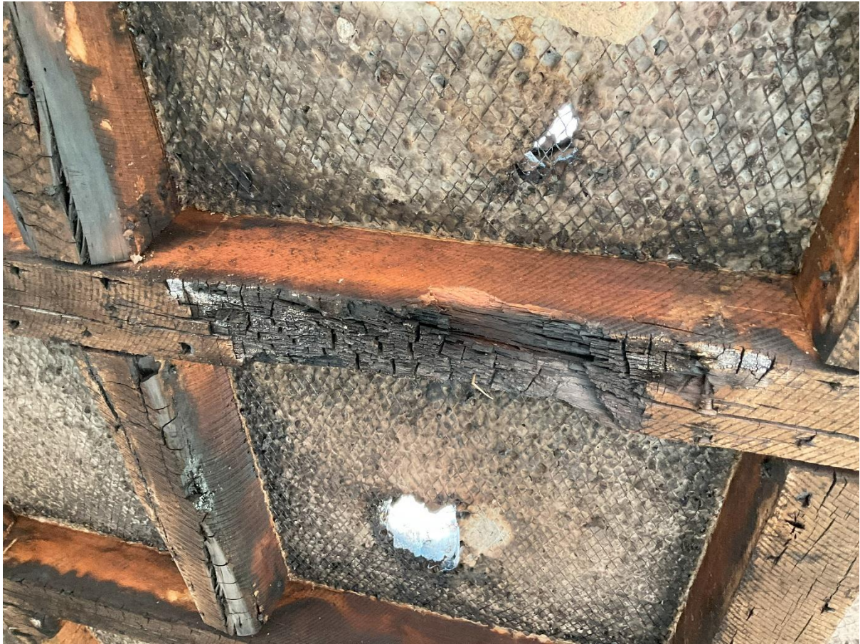
Figure D.7: Extensive timber section reduction
