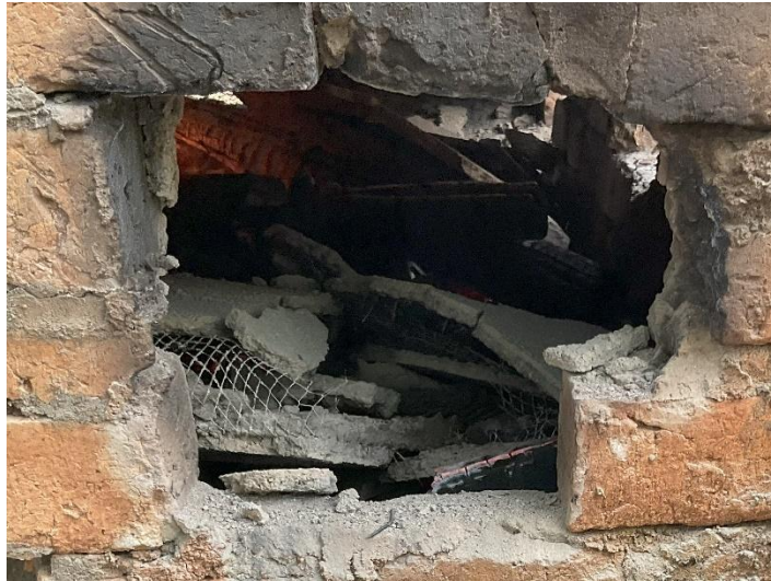
Figure 4.6: Plaster collapse in the heating phase
