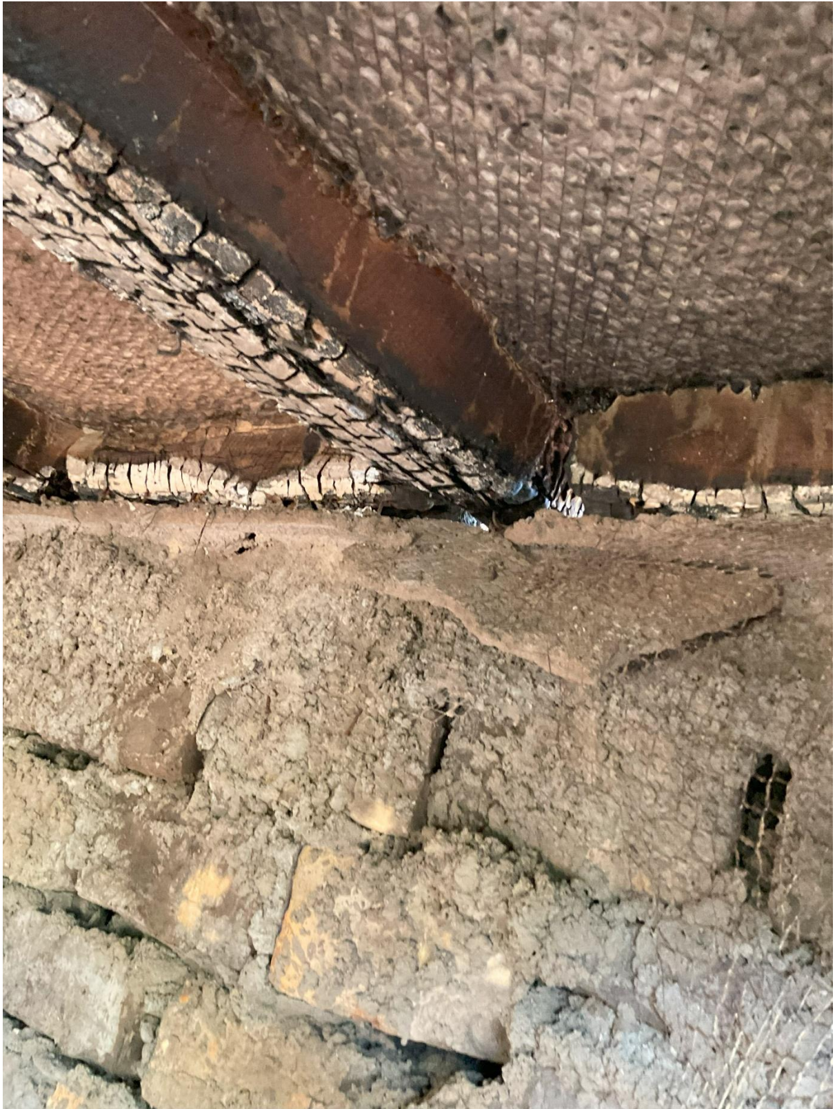
Figure D.6: Char on timber beam after cooling
