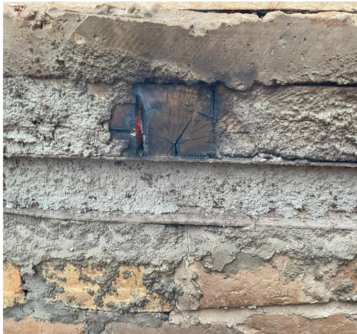
Figure 4.7: Burning timber after ignition
