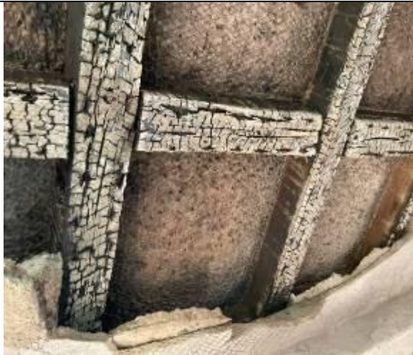
Figure 4.11: Charring of timber secondary beams
