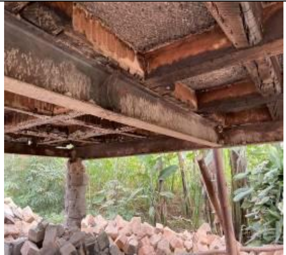
Figure 4.12: Charring of timber even where the plaster had not fallen
