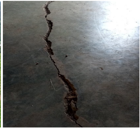
Cracks in floors
