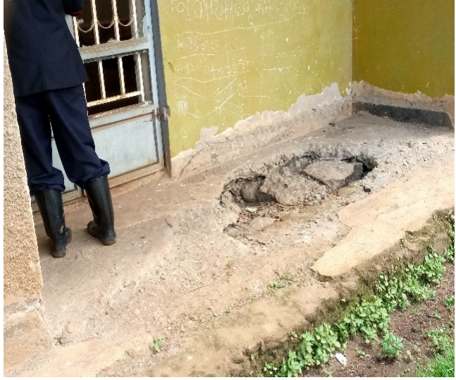
Typical floor damaged
