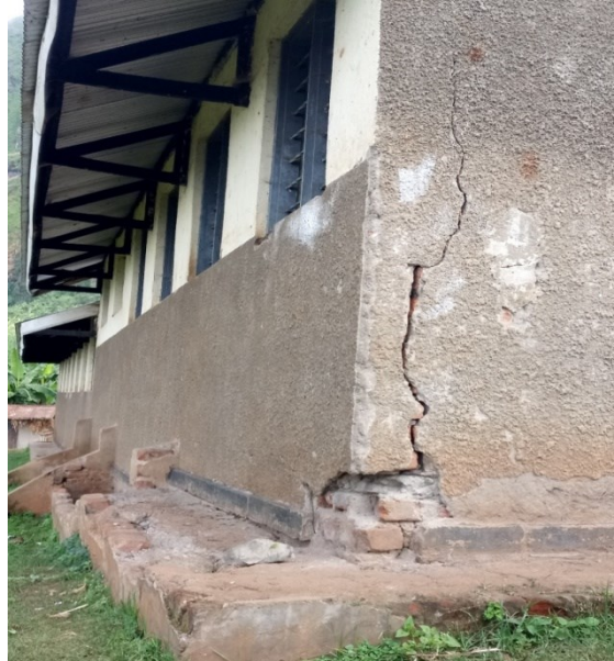
Structural Crack above in wall
