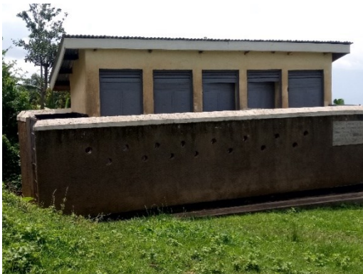
5-stance VIP Latrine
