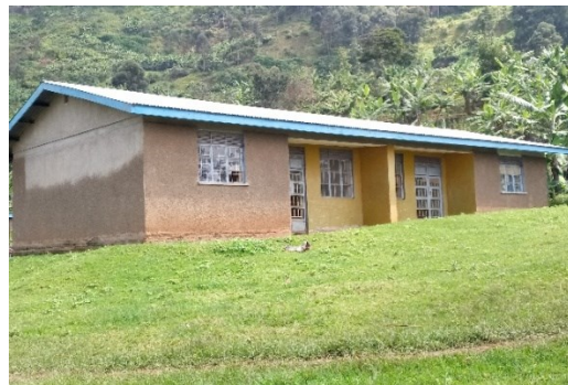
Staff House - abandoned due to defects
