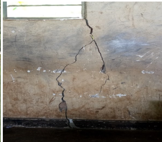
Cracks in floors
