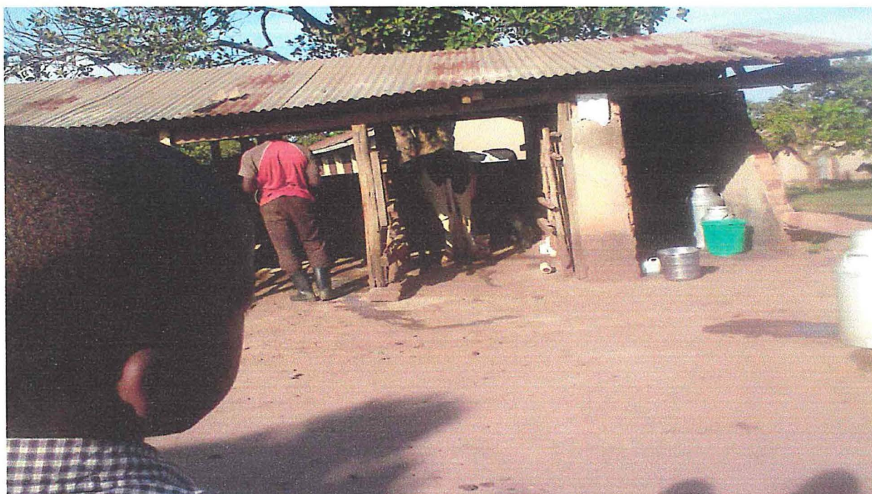
Figure 2: A dilapidated milking parlour, store and the milking equipment/tools used at KyU farm
