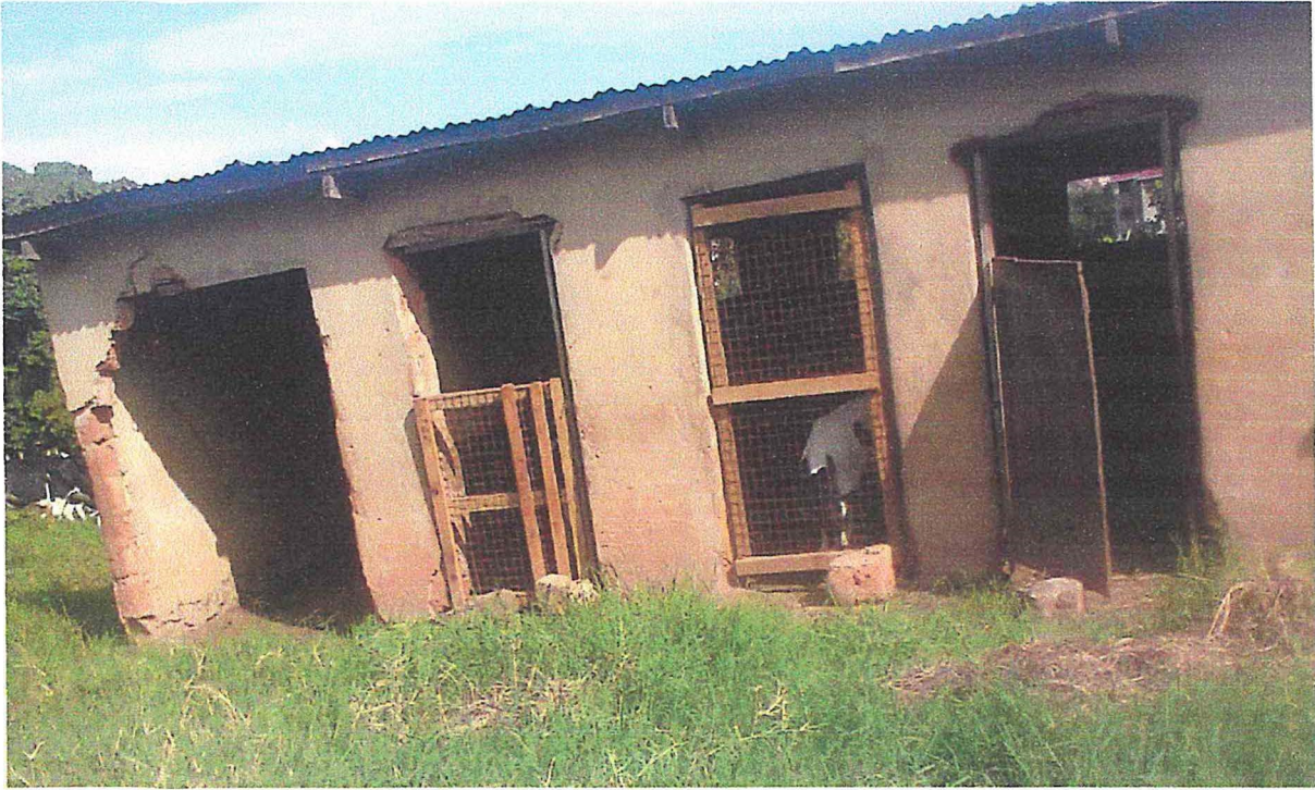
Figure 3: A dilapidated Calf Pen at KyU farm
