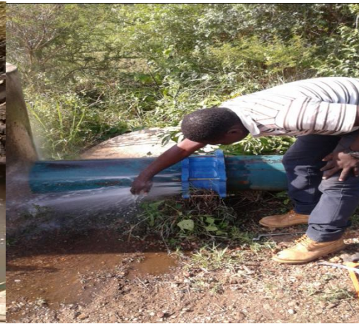
Leakage on the pipe joint
