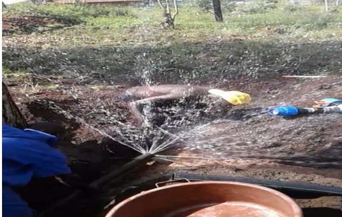
Losses from a vandalized pipe
