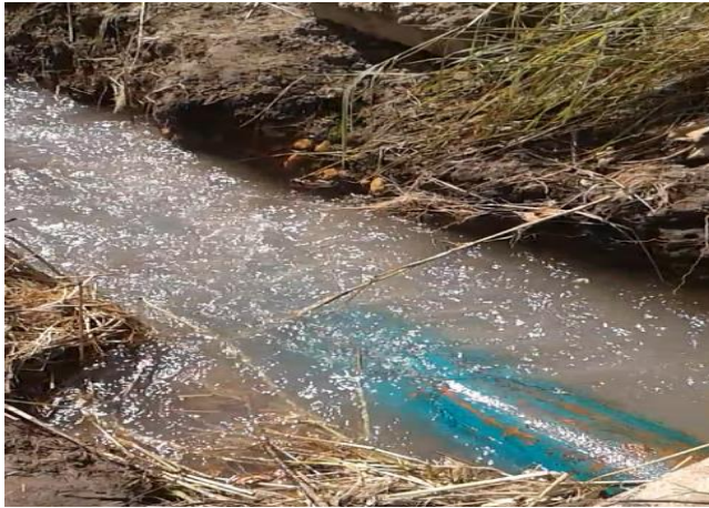
Burst on the PVC and G.I interlink
