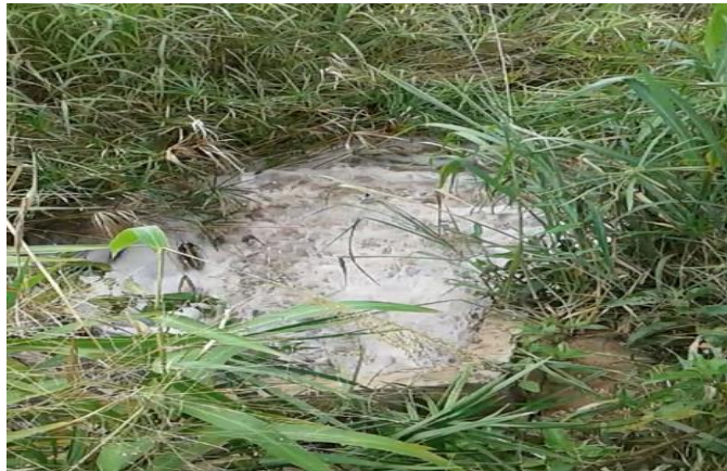
Loss from Washout
