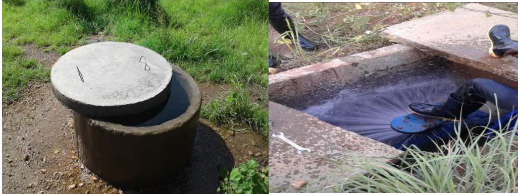
Continuous losses at the air valve
