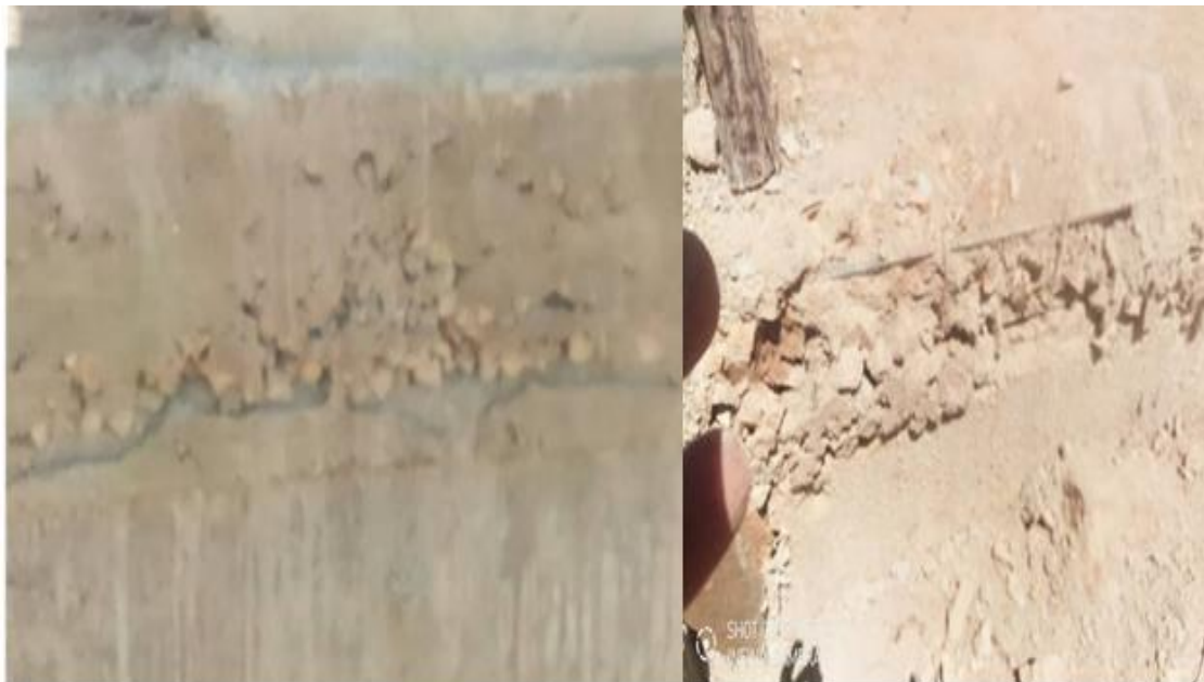
Figure 2: Maternity ward at Lwajje health III honeycombing due to poor compaction
