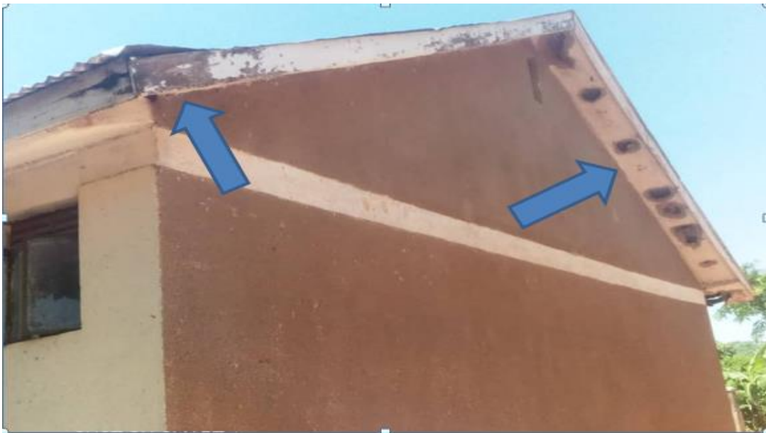
Figure 6: Staff house of Bukaali primary school of 2018 with poor construction on the eaves
