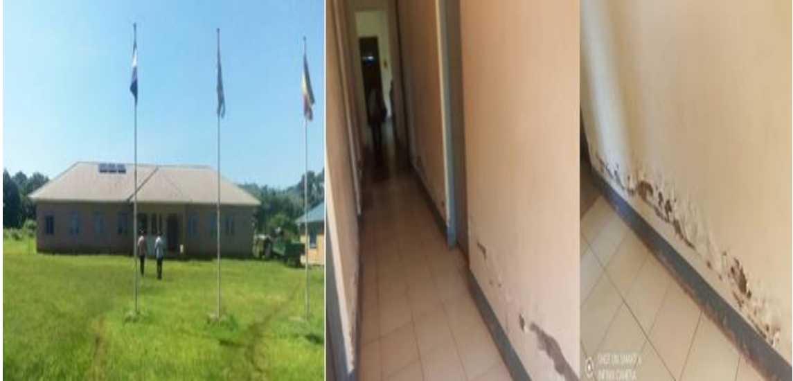
Figure 11: Water percolation into walls at Buvuma town council offices of 2018 due to poor construction
