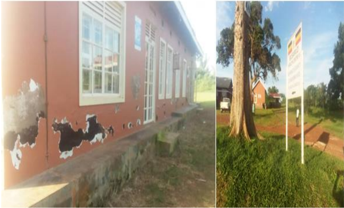
Figure 3: Busamuzi health centre III of 2020 and now the underwater penetrated in the wall due poor dump proofing
