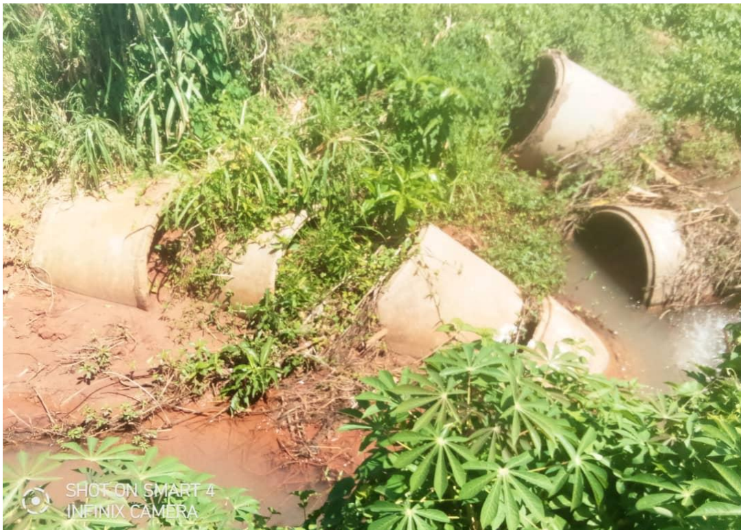
Figure 10: Culverts installed by Buvuma town council under road fund in 2019 were washed away by stormy water along Kirongo –galamo road due to poor installation.
