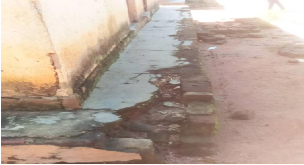
Figure 5: Staff house of Bukaali primary school had cracks on the splash apron due to poor mixes and construction
