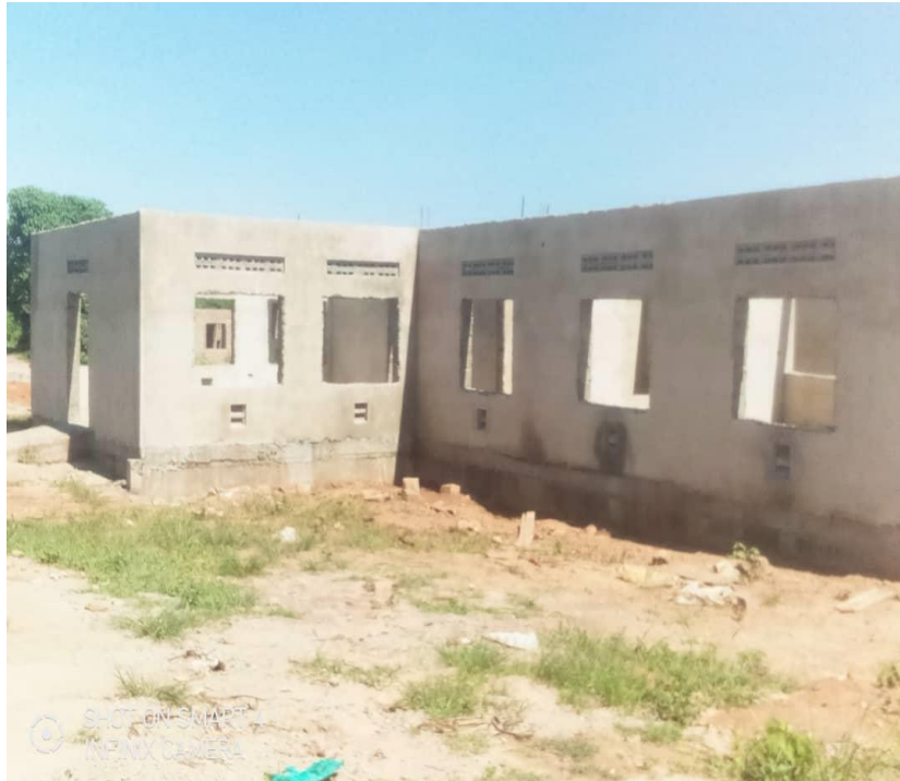
Figure 1: Maternity ward at Lwajje health III under UGIFT which was meant for financial year 2020-2021 never completed to date.
