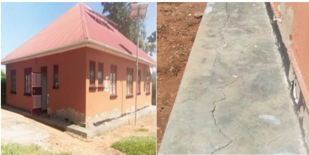
Figure 4: Buwoya Health III of 2019 had underwater penetrated in the wall and cracks on the splash apron
