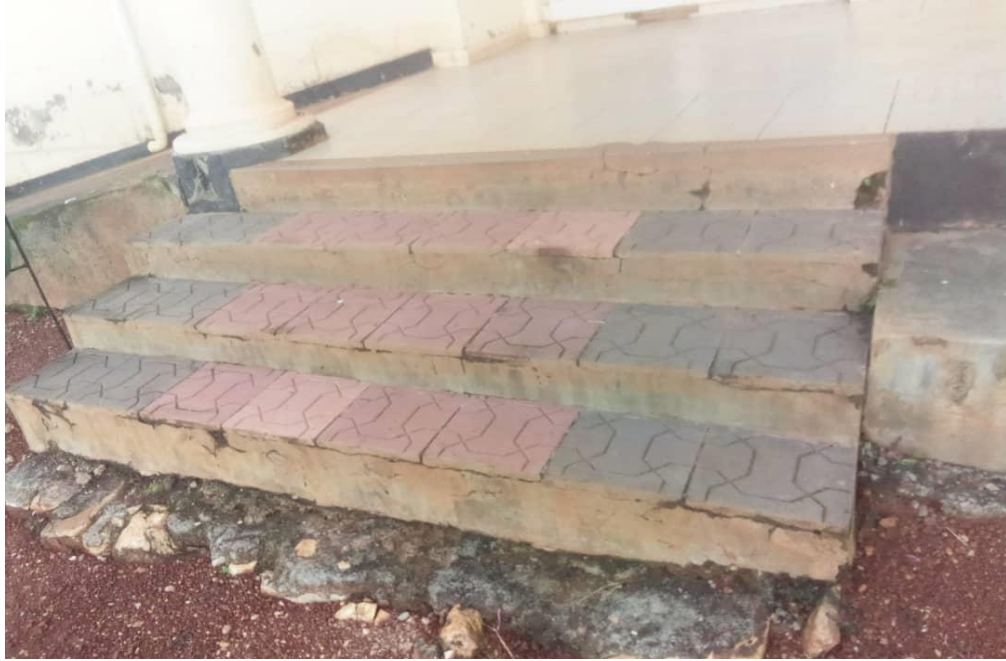
Figure 9: Peeling off concrete floor tiles on the veranda of RDC office 2017 due to poor construction
