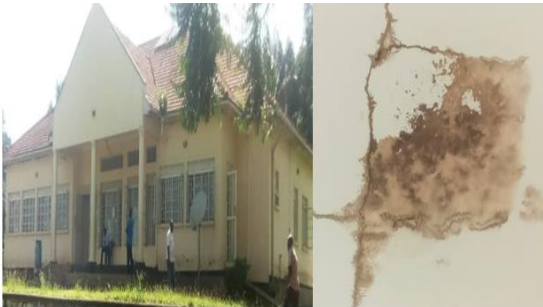
Figure 8: Linkages on the roof of the Resident district commissioner's office of 2017 due to poor roof construction
