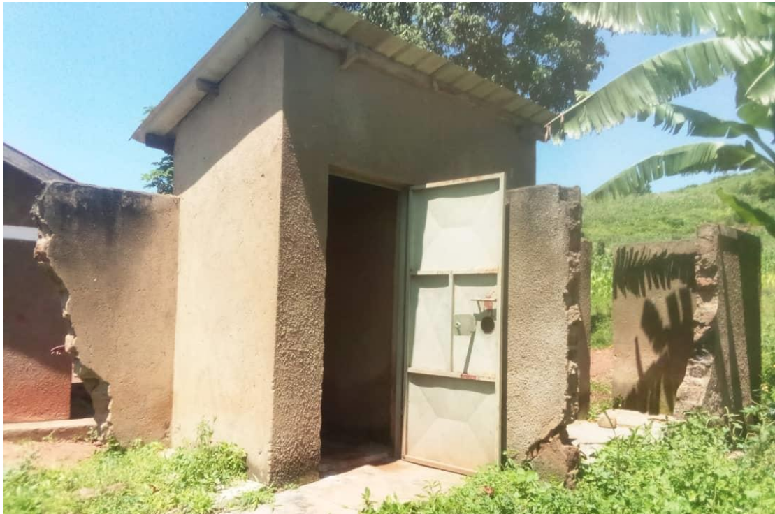
Figure 7: Collapsed toilet wall of 2017 at Buwanzi primary school due to poor construction and mixes
