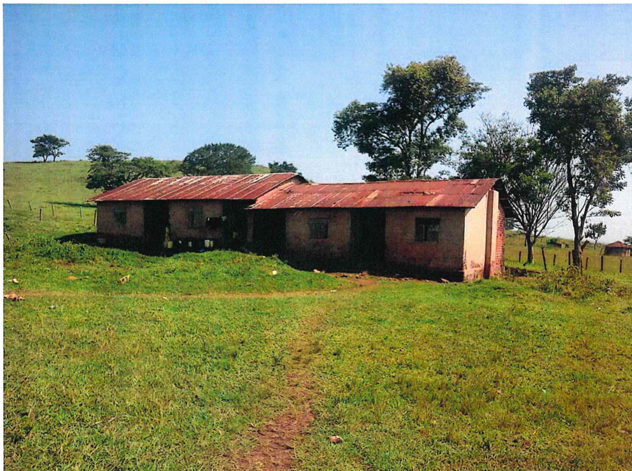
Photo 4: Dilapidated and Condemned Staff Quarters at St. Marys Kiryowa Primary School
