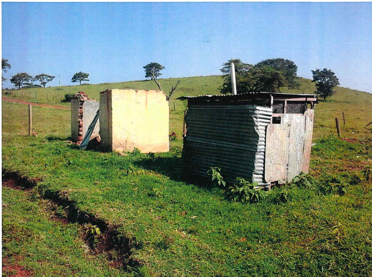
Photo 3: Poor Toilet Facilities at St. Marys Kiryowa Primary School
