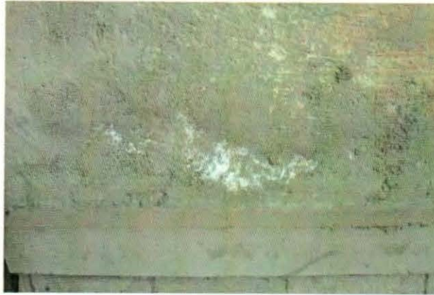
Figure 1.1 : Efflorescence on built walls
