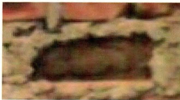
Figure 1.3 : Erosion of burnt clay brick in built wall
