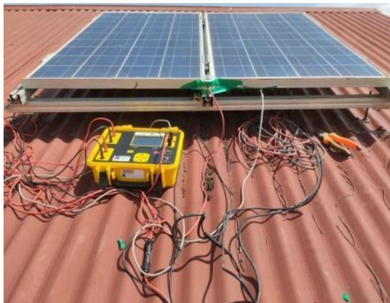
Figure 3.3: I-V Tracer connected to the modules at Orungo High School.
