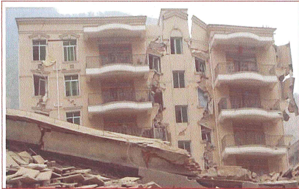
Figure 0-1: Failure in masonry infill due to seismic actions
