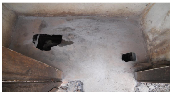
Fig. 4 A weak slab over a pit full of water with a foul smell
