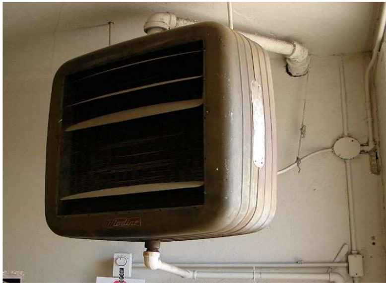
Figure 2.8: Fan coil unit (Xu & Wang, 2017)
