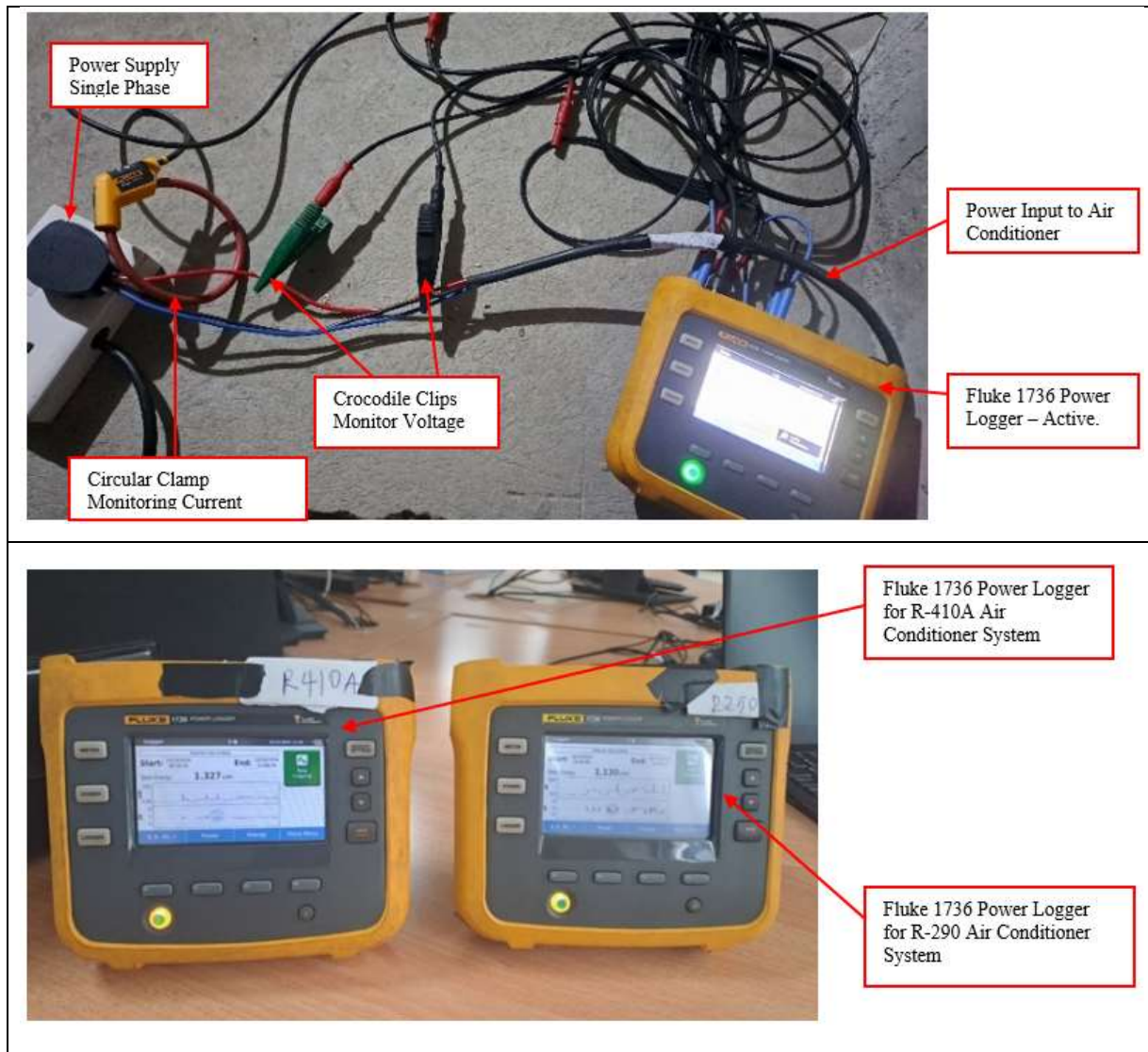
Figure 3. 5: Setup of power loggers during the experiment
