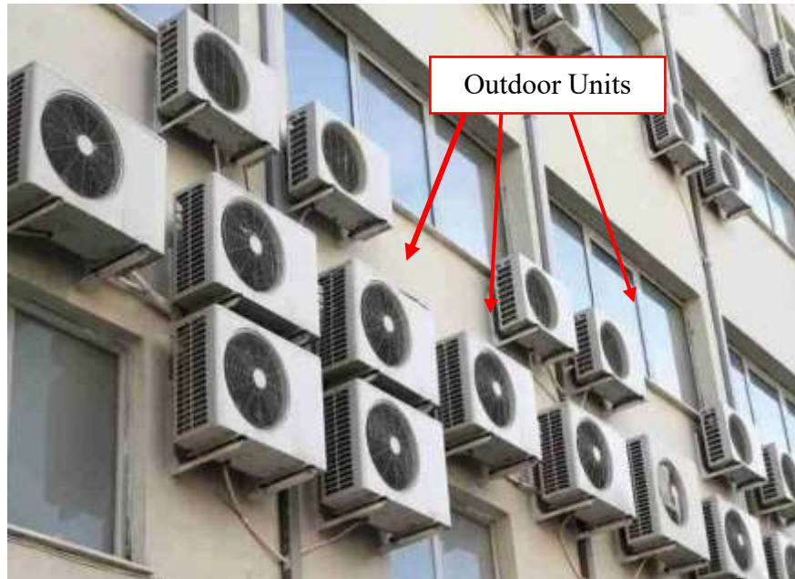
Figure 2.1: Outdoor units of split air conditioners installed for building cooling
