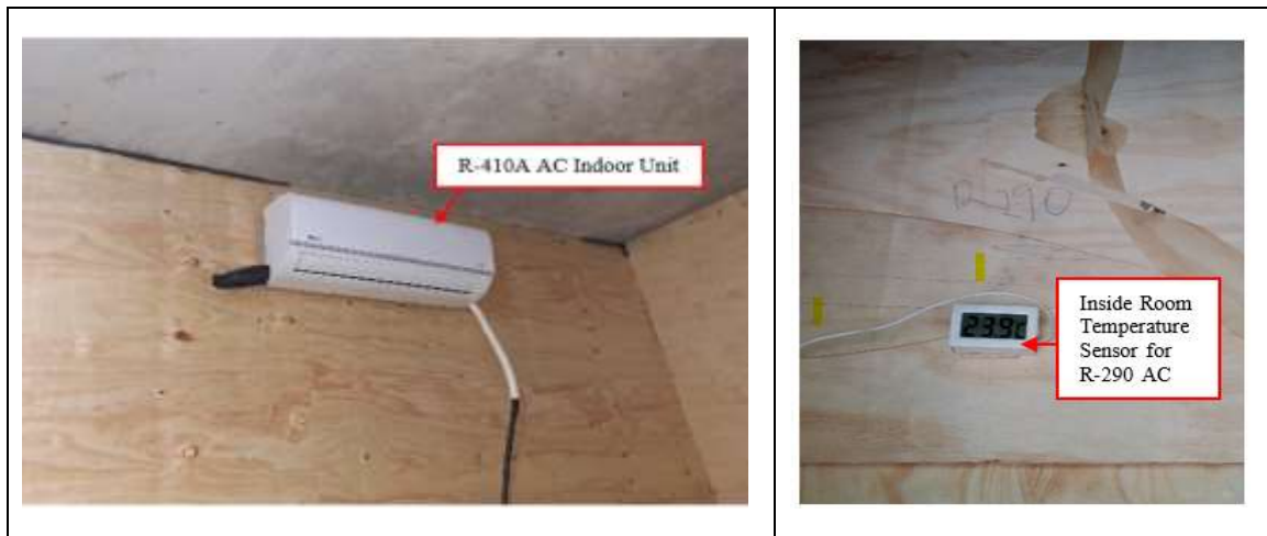
Figure 3.3: Mounted Indoor unit of one of the R-410A air conditioner and inside room temperature sensor.
