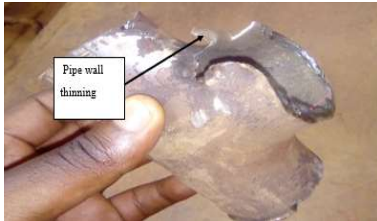
Figure 4-14. MS-tee wall thinning due to corrosion-erosion
