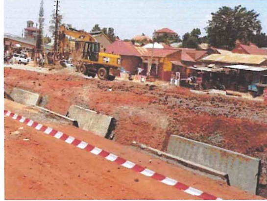
b) Encroachment of drainage reserves
