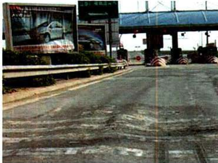
Figure 2.6: Pavement distress in China (Zou, 2017)
