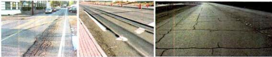
Figure 2.9: (Left) Fatigue cracking, (Middle) Rutting and (Right) Low temperature cracking (Zou, 2017)
