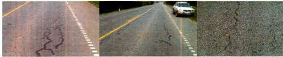
Figure 1.1: Cracking along newly completed Mbarara – Kabale – Katuna road
