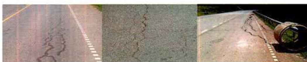
Figure 1.3: MBP – Repair of cracks MN - Shear Cracking Shear Failure and Cracking
