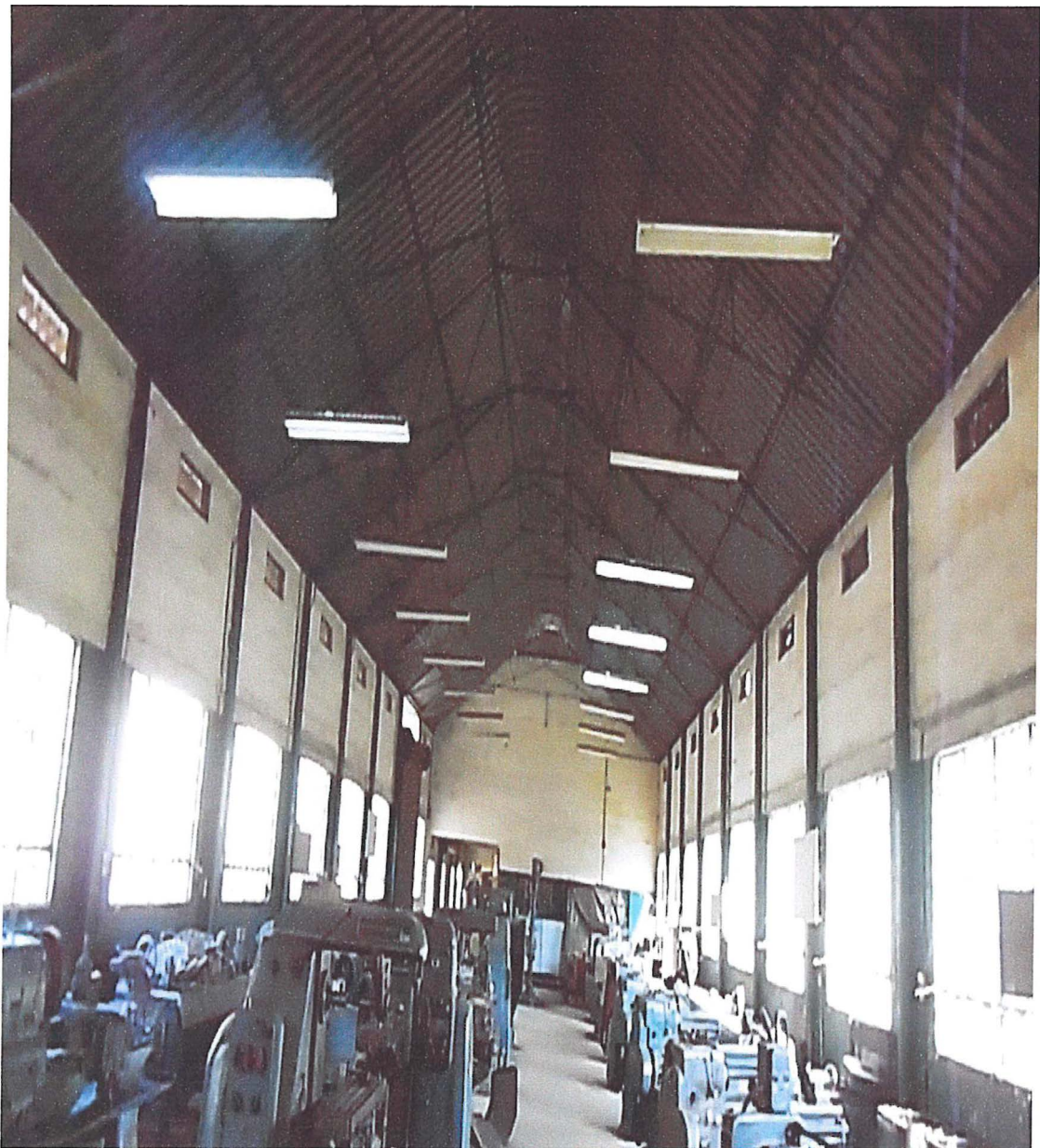
This plate the workshop walls without any warning sign
