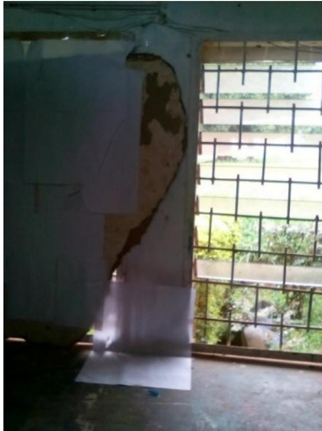
Figure 10. Broken windows in one of the exhibition rooms
