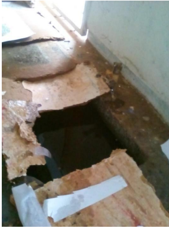
Figure 6. A malfunctioning sink in the printing studio with dirty water and environment.
