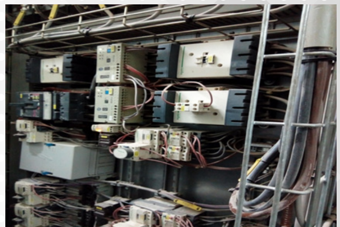
Power supply system at Ntake Bakery and Company Limited
