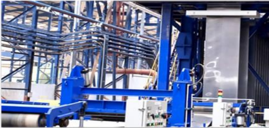
Figure B-4 : Galvanizing of the sheet in process- galvanizing bath (on site pictures)
