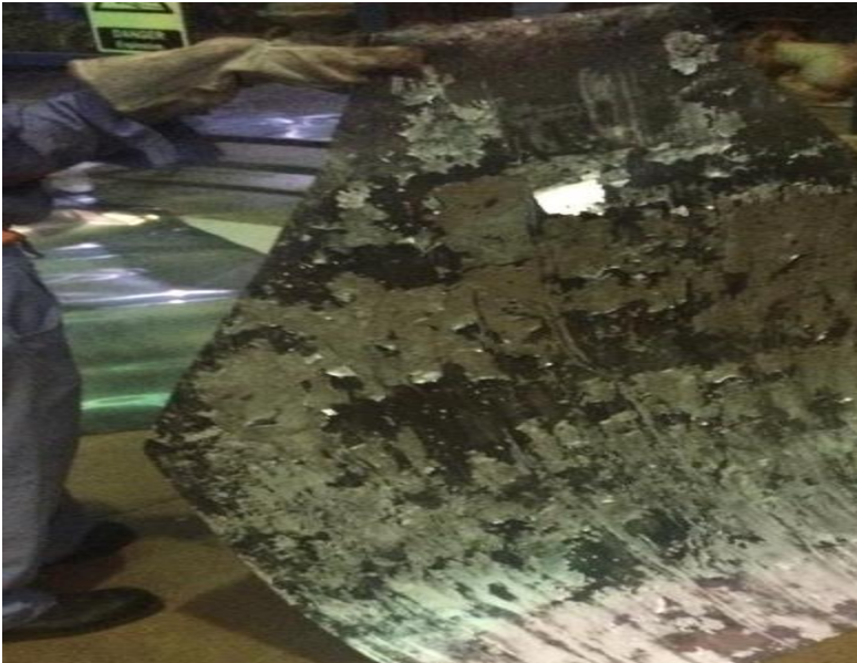
Figure B-11 : Damaged sheet (burnt and black spots) (on site pictures)
