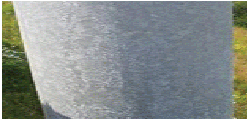
Figure 2-17 : Light Wet Storage Stain (AGA, 2016)
