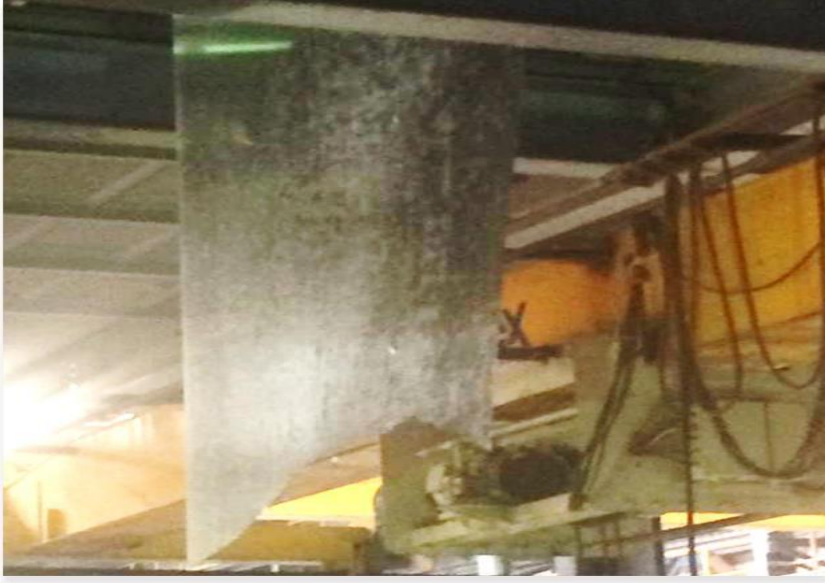
Figure B-13 : Torn galvanized sheet at the galvanizing bath (on site pictures)
