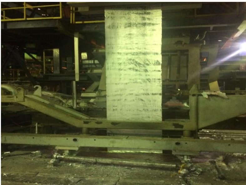
Figure B-12 : Rough Surface condition on the Sheet (on site pictures)
