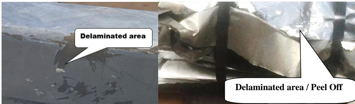
Figure 4-5 : Delamination's and peel offs (on site pictures)
