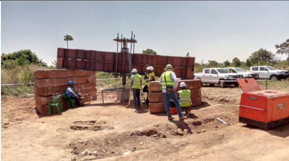
Equipment setup for the Test at B103/5 (KL 30)
