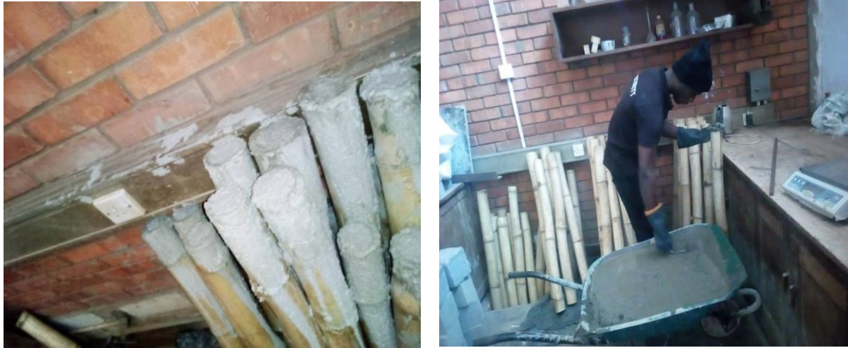
Figure 3.8: Casting designed concrete mix into the hollow bamboo. Left: Cast concrete setting in the hollow bamboo before curing.
