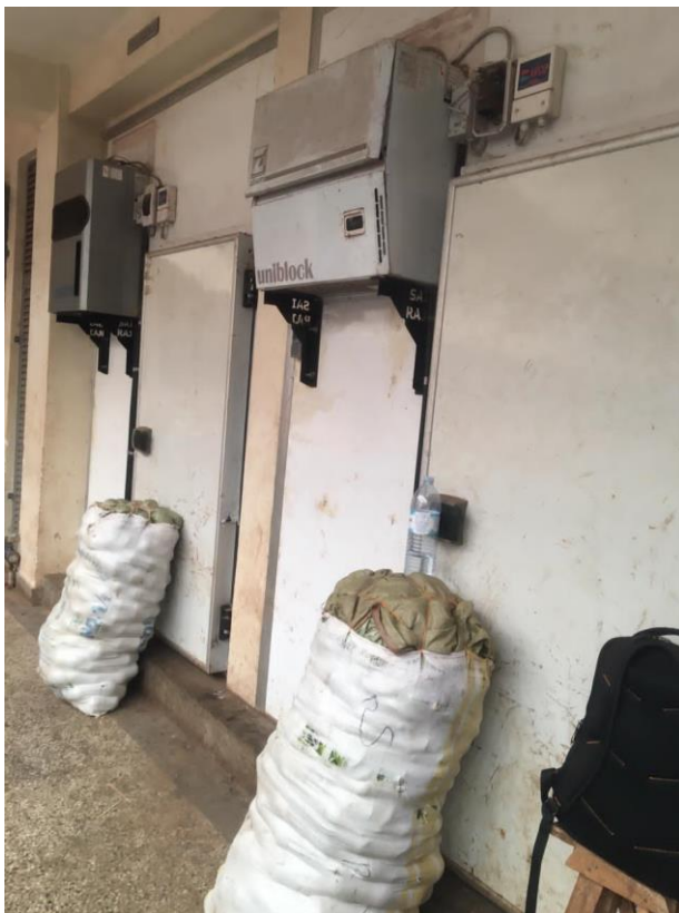
A walk-in cold room at one of the central markets
