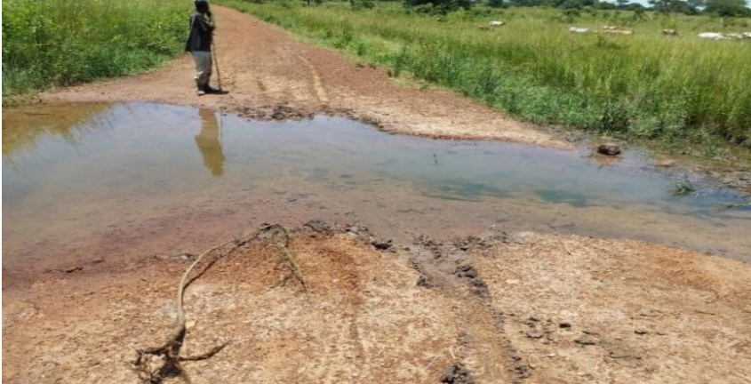
Figure 1. 1: Poor drainage along Usuk-Ongongoja road which poses threat to the quality of roads in Katakwi district
