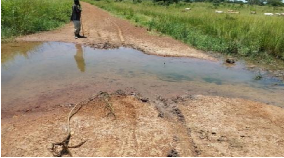
Figure 4. 6: Poor drainage along Usuk-Ongongoja road
