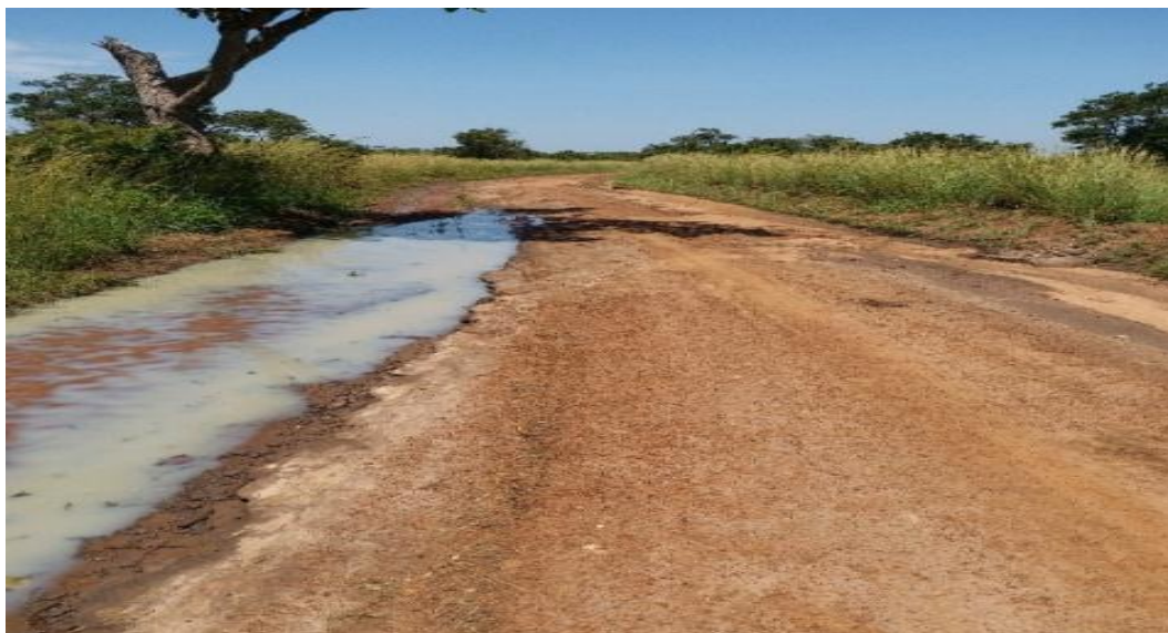
Figure 4. 8: Poor drainage along Getom-Toroma road
