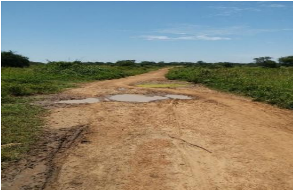
Figure 4. 7: Poor drainage along Ngariam-Palaam road
