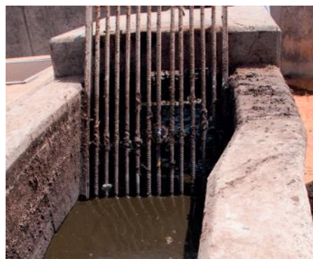
Figure 2. 1: Niayes faecal sludge treatment plant screening in Dakar, Senegal
