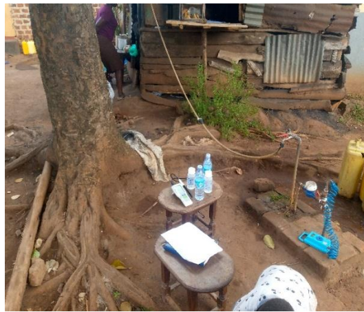
Figure 3.3: pressure Logger installed at the customer's meters to measure pressure
