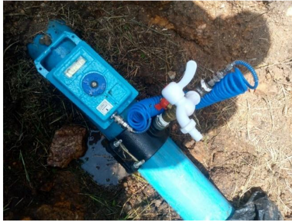
Figure 3.4: point created on the DN100 pipeline with a pressure logger installed and tap point to collect water sample
