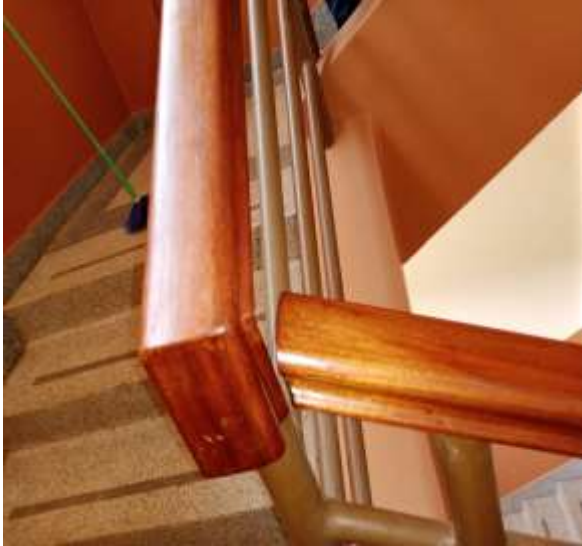
Photograph 1: Showing broken handrail
