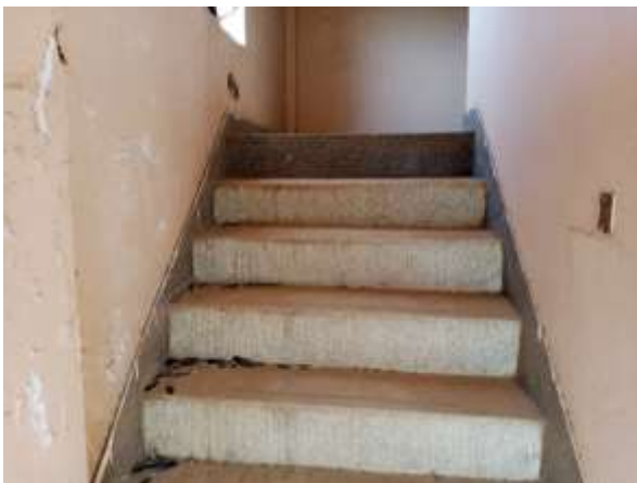
Photograph 8: Showing stair flight with uneven risers
