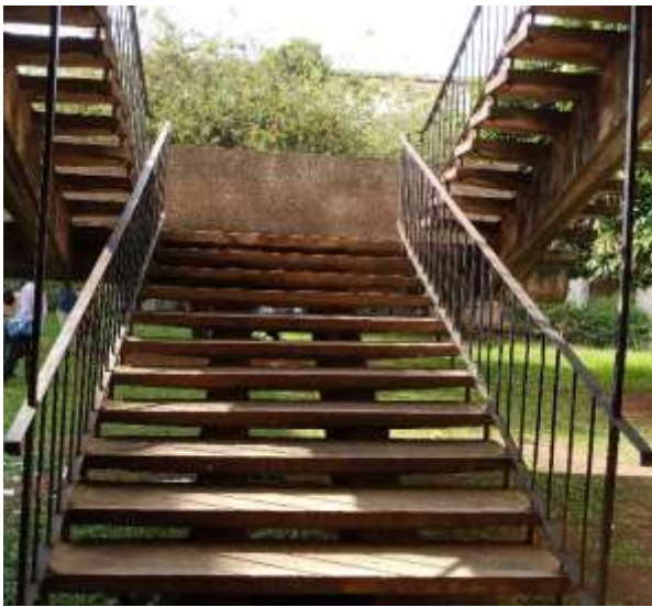
Photograph 13: Showing stair flight with open risers
