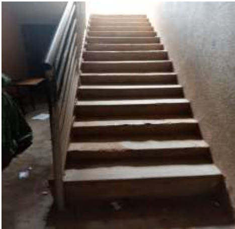
Photograph 6: Showing uneven steps
