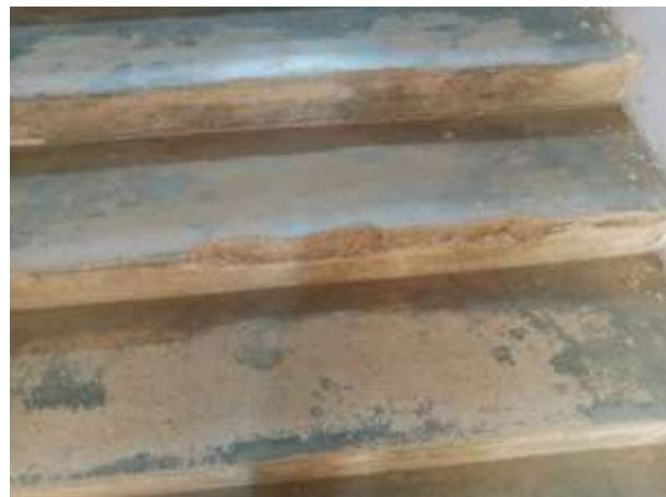
Photograph 7: Showing steps with broken edges
