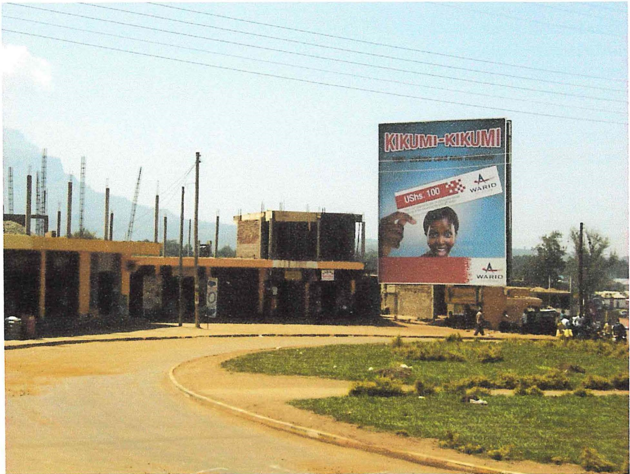
Figure 4.27: New constructions at Mbale Bus Park in South Central Ward in Industrial Division.
