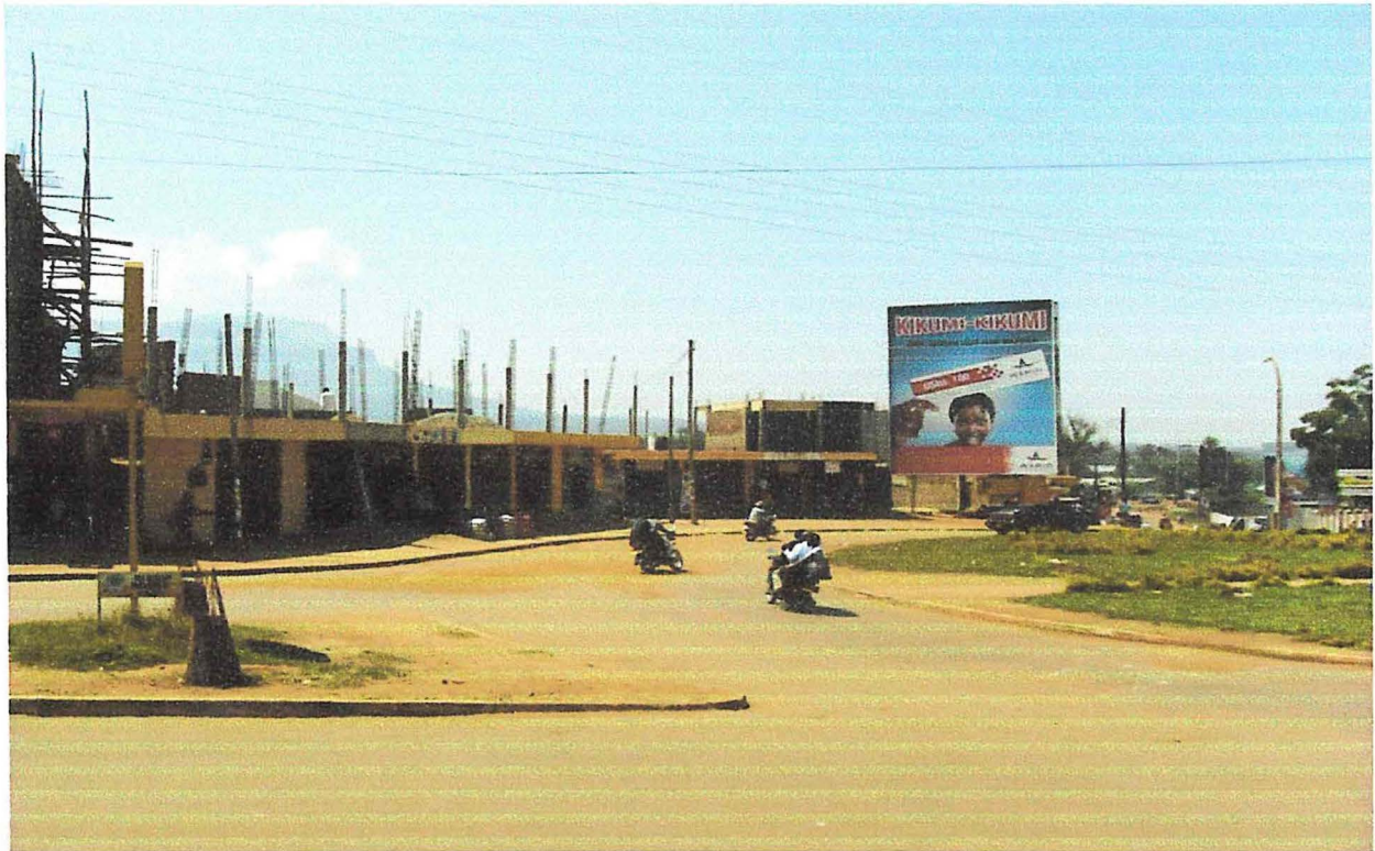
Figure 4.20: Building under construction at Mbale Bus Park in South Central Ward in Industrial Division
