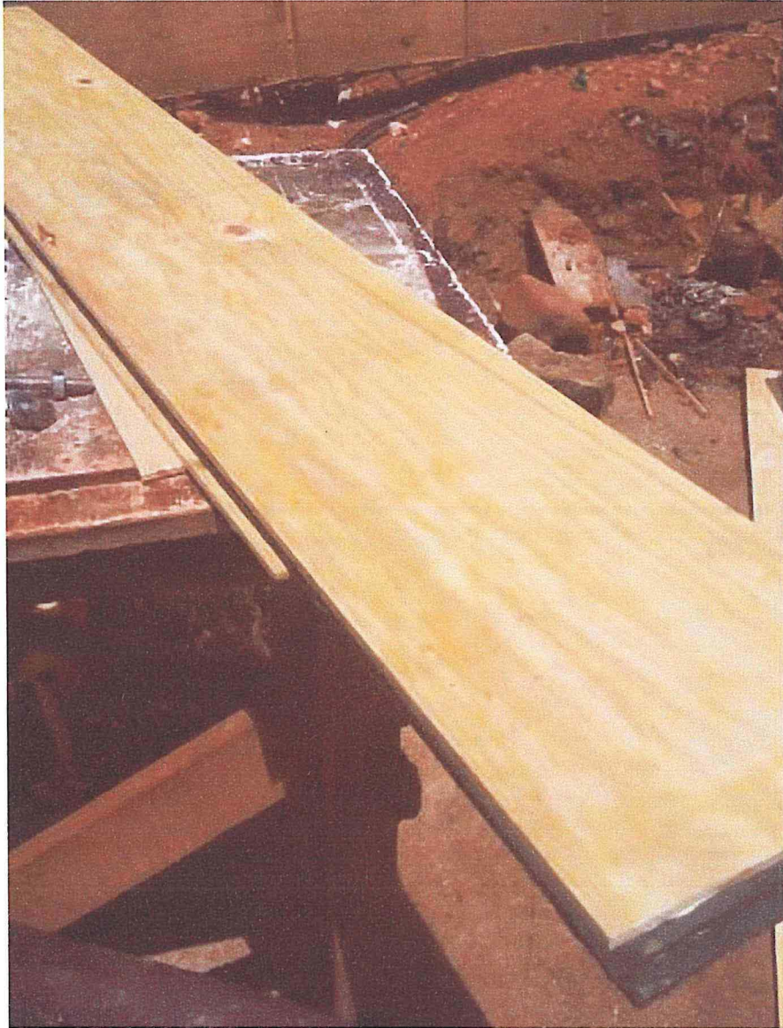
Figure 4.5.9: 6mm thick safety rail ply being ripped with a power saw. Source: Photograph by the Researcher, 2018
