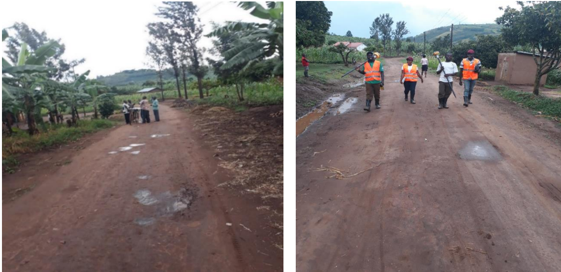
Figure 4. 12: Roads in Kanywamaizi parish exposed to the dam flood
