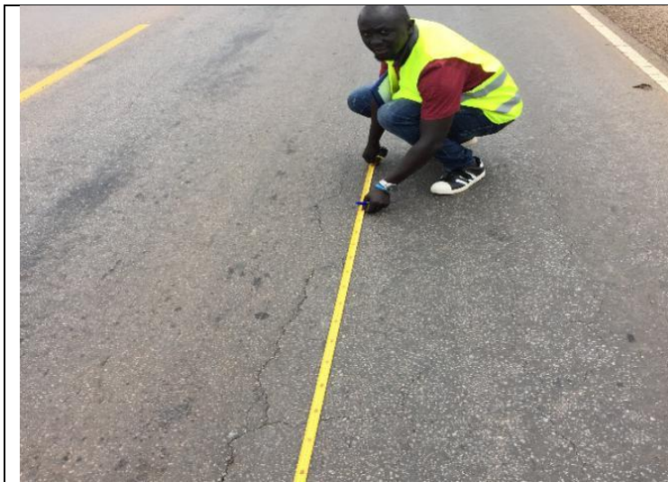
Measuring the length of longitudinal cracks from Km 98+640 to Km 98+890 –
