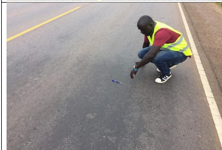
Aggregate loss from bitumen from Km 99+710 to Km 99+870 –
