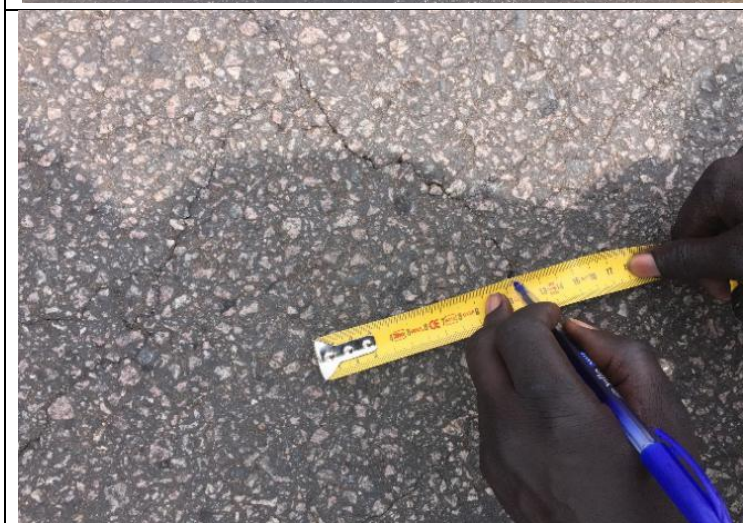
Measuring the width and depth of Alligator cracks at Km 101+330 and Km 101+490
